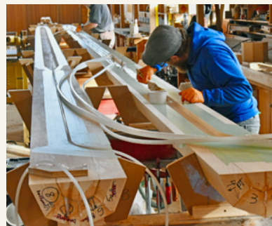
The mast had solid blocking at both ends. Conduits for wires were installed before the two halves were glued together.
