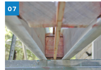
07 Good view of the lower angled fiberglass edge.
