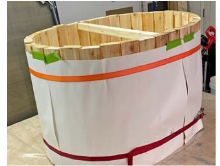
Ratchet straps were used to draw the vertical strakes together while the epoxy cured.
