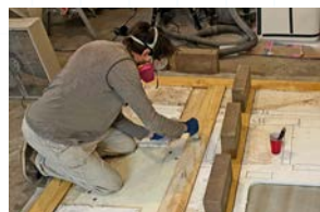
Applying a neat coat of epoxy before bonding the plywood to the fiberglass wall panel.
