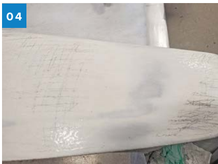
04 The high areas have been sanded down into old fairing compound and fiberglass. The remaining pencil lines indicate the low areas where the new fairing compound needs to be applied.
