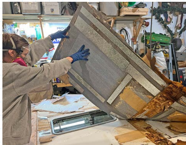
Peeling back the lauan panel seeing the true extent of the water damage.
