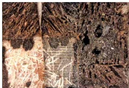
Water seeped into the swim platform causing extensive rot in the balsa core.
