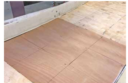
The plywood was cut into smaller sections to make it easier to install.
