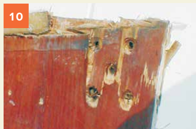
Rotted plywood should have the compressed section replaced.
