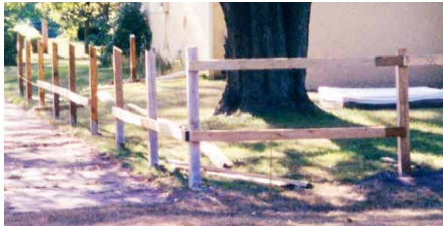
The epoxy-encapsulated posts were set in concrete and tied together with stringers.
