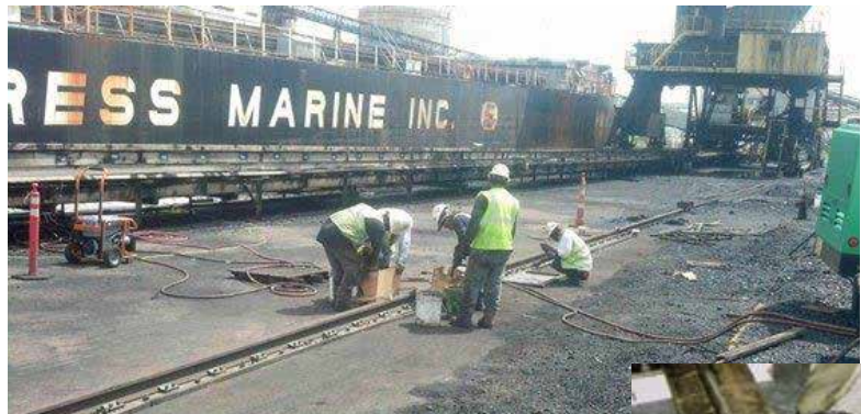
A new crane rail being installed at a power company coal pier.
