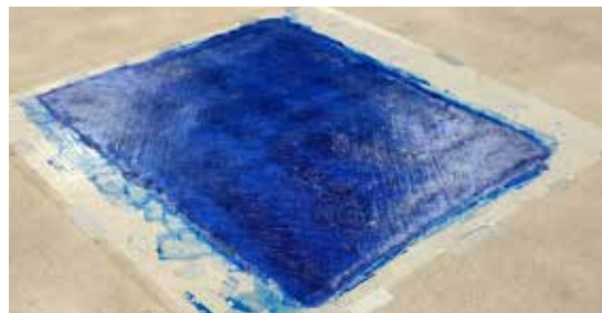
The shop floor, covered with plastic, was a great location for laying up a large flat panel.
