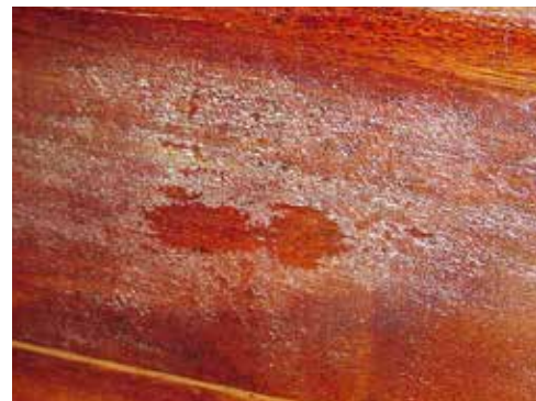
The crazing pattern and underlying shiny varnish. It's on the side, near the transom in an area of high UV exposure.
