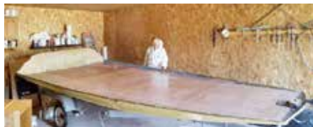
8mm Okoume bonded with WEST SYSTEM Epoxy on both sides, and tabbed to the edge of the hull
