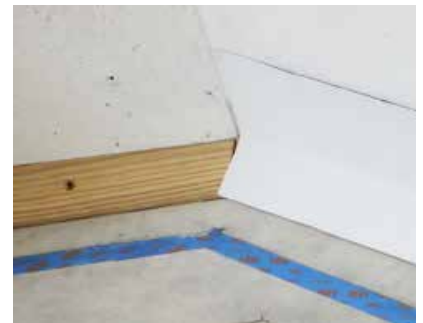
The wood strip on the left is a 45° beveled piece ripped from "two by" PT lumber. The right is six inch wide "peel and stick" flashing membrane.
