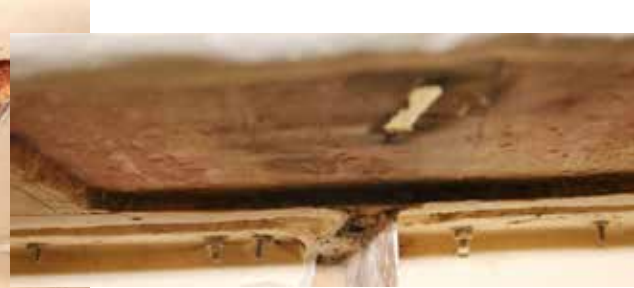
The rotted core removed between the two skins at the hull/deck joint.
