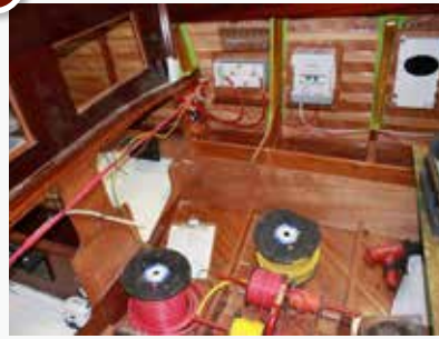
The engine room is wired before the engines are set. Van Dam does all wiring to ABYC standards with team members who are ABYC certified.
