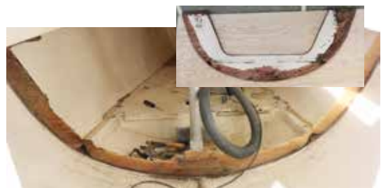
The bulkhead has been removed and the tabbing that was on the back side was left in place. Inset, the intact bulkhead that was removed.
