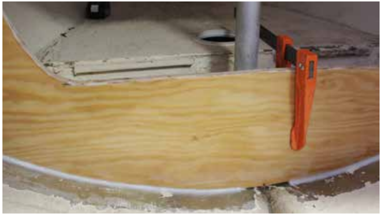
The new bulkhead clamped to the tabbing from the old bulkhead to hold it in place, and the new fillet applied.
