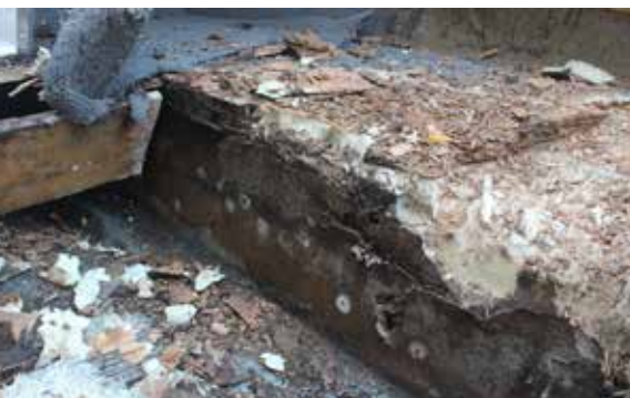
Rotted stringer and damage done to the flotation during wood removal
