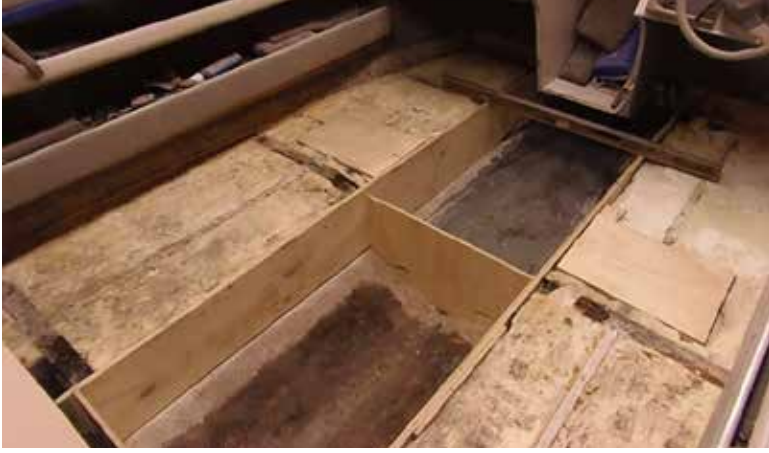
The plywood stingers and bulkhead have been dry fit. The backing panels for the butted plywood seams are set into the foam.
