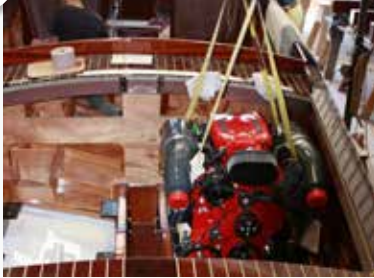
With the shaft logs installed and the bilge area painted white, the first engine is lowered into place and set on custom aluminum mounts.
