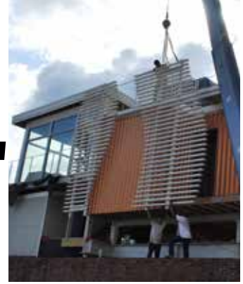
Cover Photo: Installing some of the assembled FRP louvered panels on the rooftop residence
