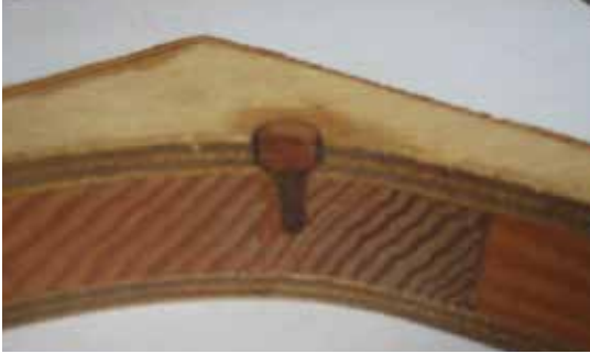
Note cutaway of hole and plug how all the end grain that the screw exposes is protected with epoxy.
