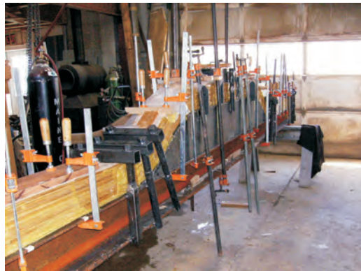
Left —Application of G/flex 655. A thin coat was squeegeed onto one surface and a thicker coat was applied with a notched trowel to the other mating surface.
