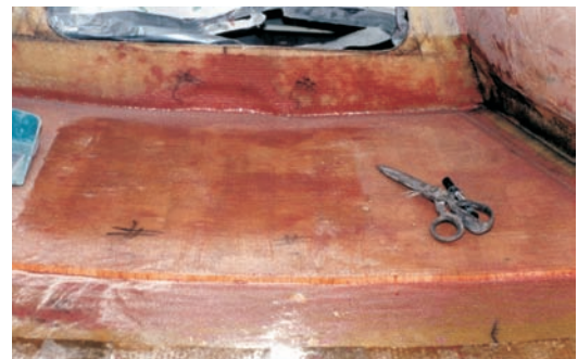
New balsa core and fiberglass skin were installed in the damaged areas.
