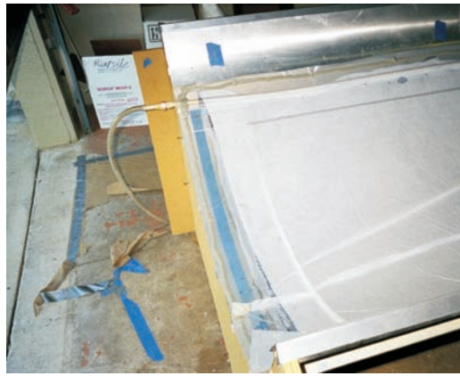
A panel curing under vacuum. The panel was built of ½"-thick Divinycel foam between layers of 6 oz carbon fiber cloth laminated with WEST SYSTEM® Epoxy.
