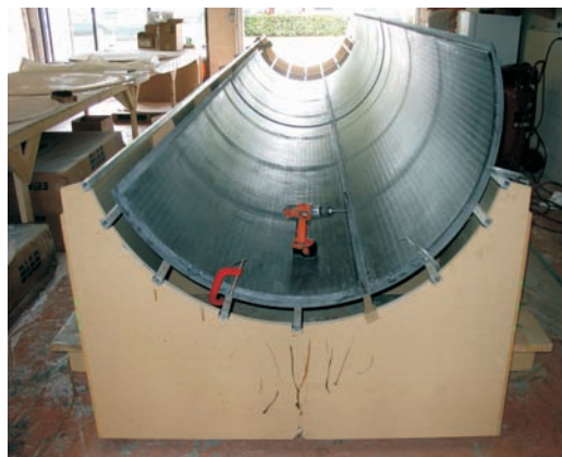
Finished panels being prepped for final assembly. The first panel joint was held in place with Cleco fasteners onto a stringer after the sheet metal had been removed.
