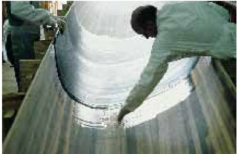
Applying unidirectional carbon fiber to the inside of Adrenalin's cedar strip hull.
